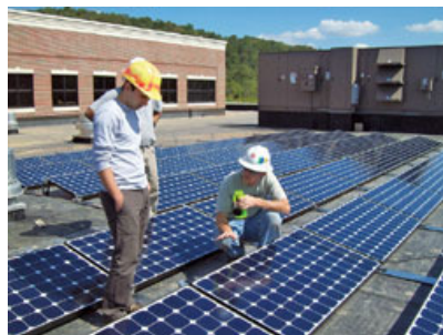
This 192-module Sunpower system atop a health clinic in Athens, Ohio, should produce
